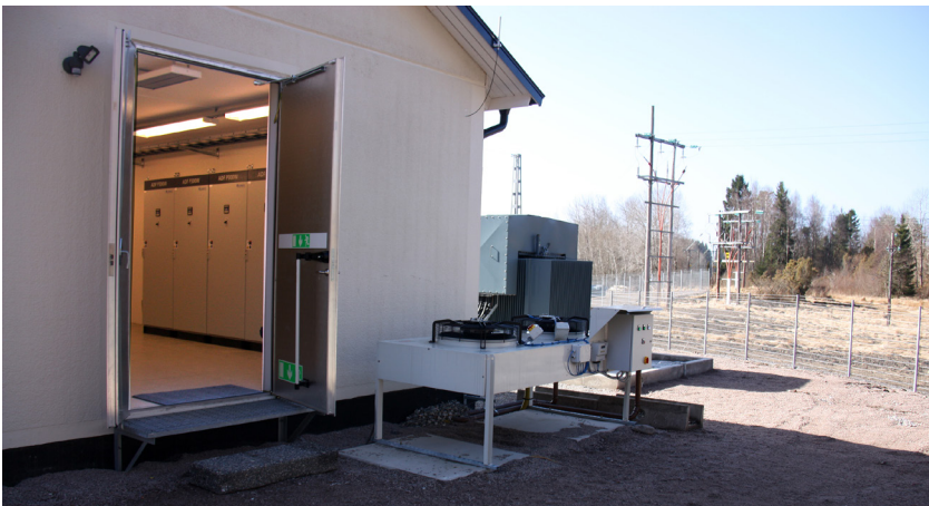
ADF STATCOM installation at the Fortum wind farm in Kville, Sweden.
